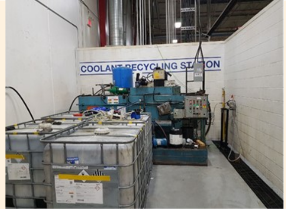
In Ancaster, Canada, the site reviewed its onsite coolant recycling programme and determined that it could reclaim more coolant, saving of 38,000 litres of coolant concentrate and 450,000 litres of water a year
