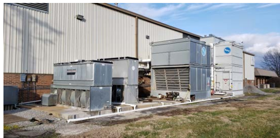
Maintenance work and improvements to chillers and other HVAC systems resulted in a 43% reduction in water consumption from FY19/20 to FY20/21 in Springfield, USA
