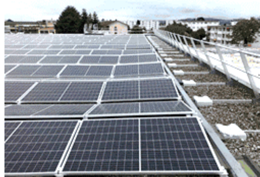
In Murten, Switzerland the Group installed 900m 2 of photovoltaic cells on the roof of the factory, generating an estimated 123 MWh per year.
