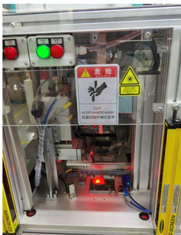
Laser marking equipment installed in Wuxi, China to replace ink marking with solvents
