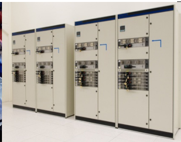
Building Automation & Security
