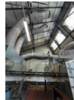
Refrigerated heat exchangers installed in our site in Saint Remy, France
