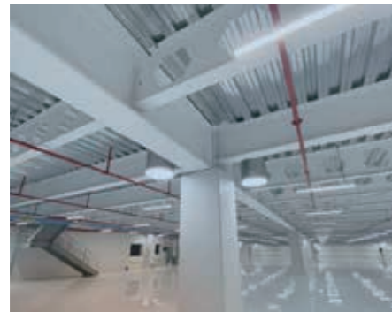
Solar tubes installed in our site in Zacatecas
