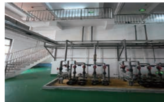
Wastewater treatment facility in our site in Jiangmen, China
