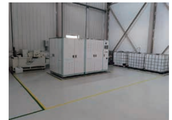
Wastewater treatment facility in Changzhou, China
