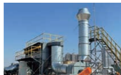
Air emission treatment facilities at our site in Shajing, China
