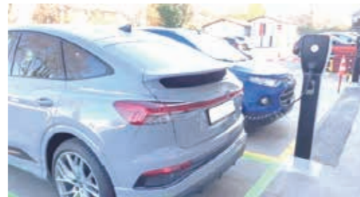
Electric vehicle charging station at our site in Murten, Switzerland
