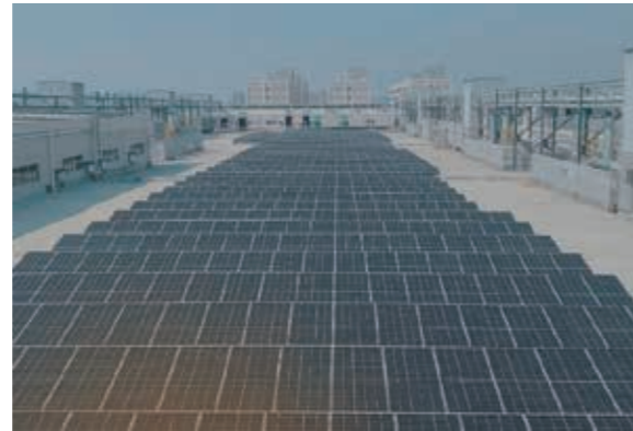
Solar panels installed in our site in Jiangmen in 2022
