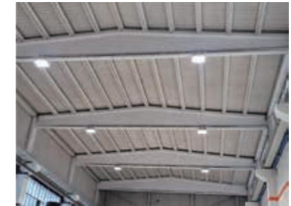
LED lights equipped in our site in Asti, Italy
