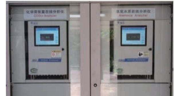
Wastewater monitoring devices in Shanghai, China
