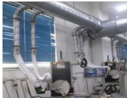
Upgrade of grinding-dust collection system
