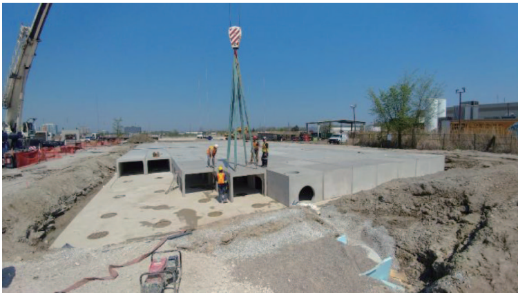
Construction of underground storm water collection and pollution prevention system in Mississauga, Canada
