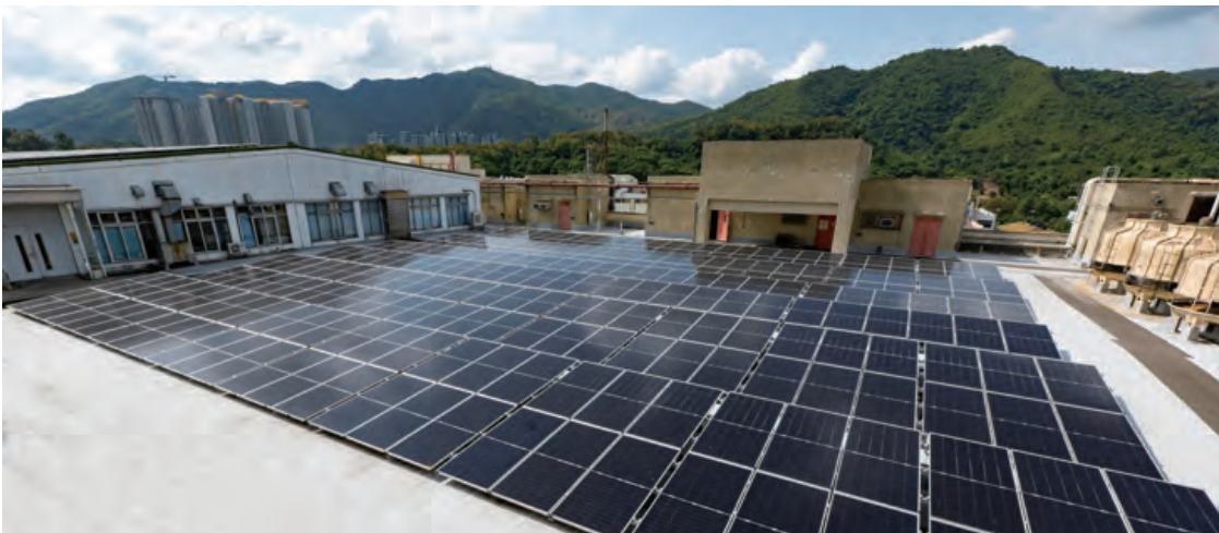
Solar panels installed in our manufacturing plant in Hong Kong in 2022
